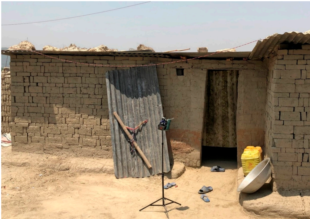
Figure 1. Typical construction of brick workers' homes sampled in this study. Construction consisted of dirt floors and un-mortared brick walls. Tin roofs were constructed by placing bamboo or wooden poles across the top of the walls, with sheet metal placed on the poles. Rocks, bricks, soil, and other heavy objects were used to hold the sheet metal in place. Indoor samples were collected by attaching PM 2.5 and temperature/relative humidity instruments to tripods as shown. Tripods with the attached instruments were placed inside the home during the entire sampling period. Abbreviation: PM 2.5 , particulate matter with an aerodynamic diameter less than 2.5 \mu\text{m} .
